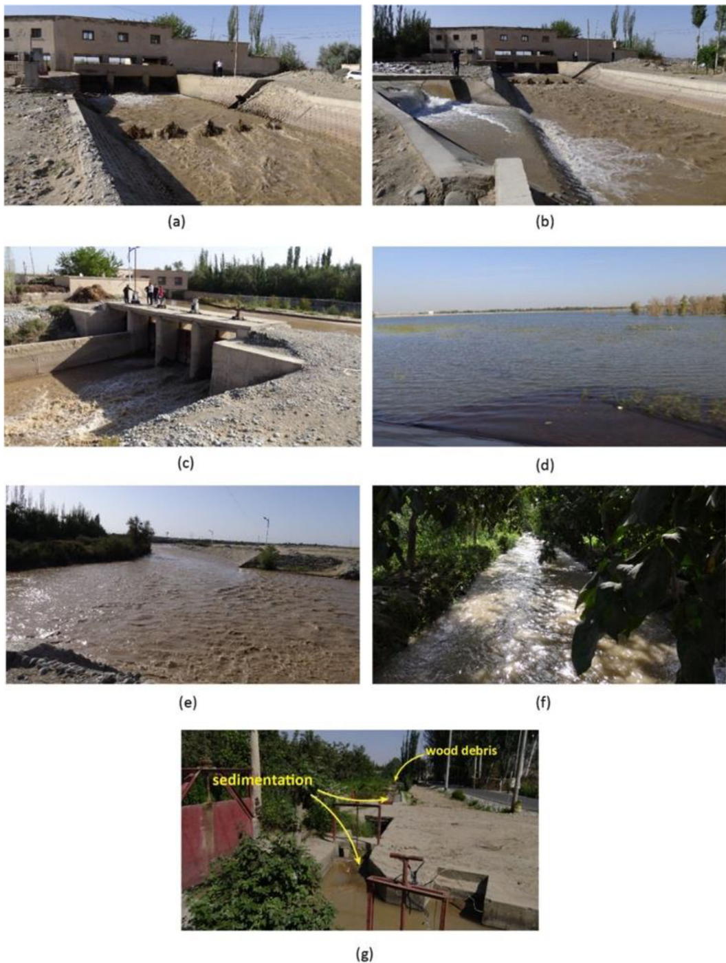
Fig. 1 Cele gate and canal system (2017). (a) Outflow at gate 1 into main Cele canal channel. (b) Inflow from Cele reservoir into main canal channel. (c) Cele River in background with outflow through gate 1 side structure toward Cele reservoir. (d) Cele reservoir. (e) Overflow of Cele River across submerged broad-
